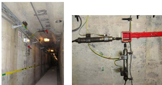
Fig. 3. A typical control gallery of a water damming structure
