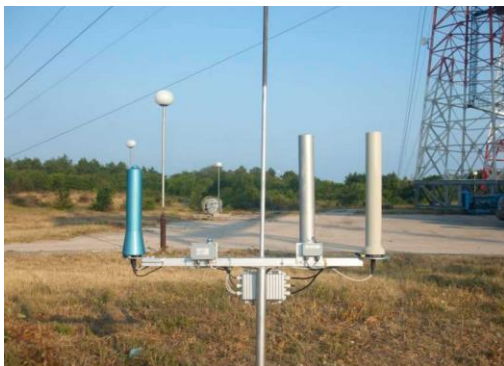
Figure 4: Photo of the upgraded sensors on an LMS. On the left is the spectrometry probe, in the middle is the start and on the right is the new dosimetry probe
