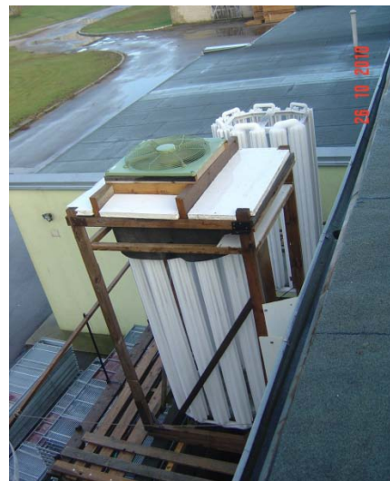
Fig.2. Ventilator above the heat pump evaporator
