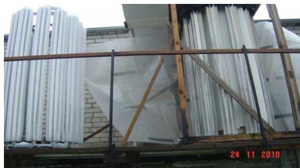
Fig.4. The evaporator block with opened screens after thawing
